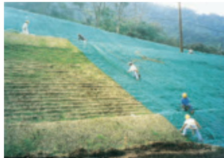
Deployment of Landlok TRM on a steep slope adjacent to Hawaii DOT H-3 project.
